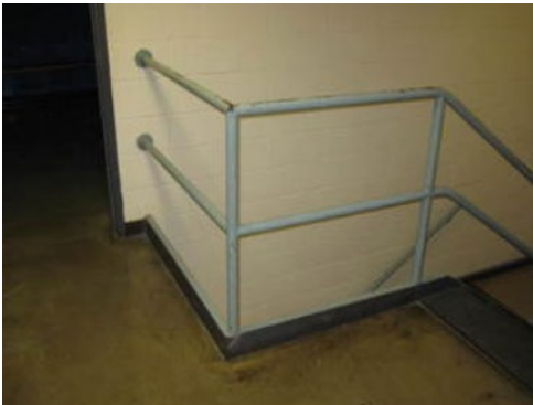
Guard/Handrail not code compliant
