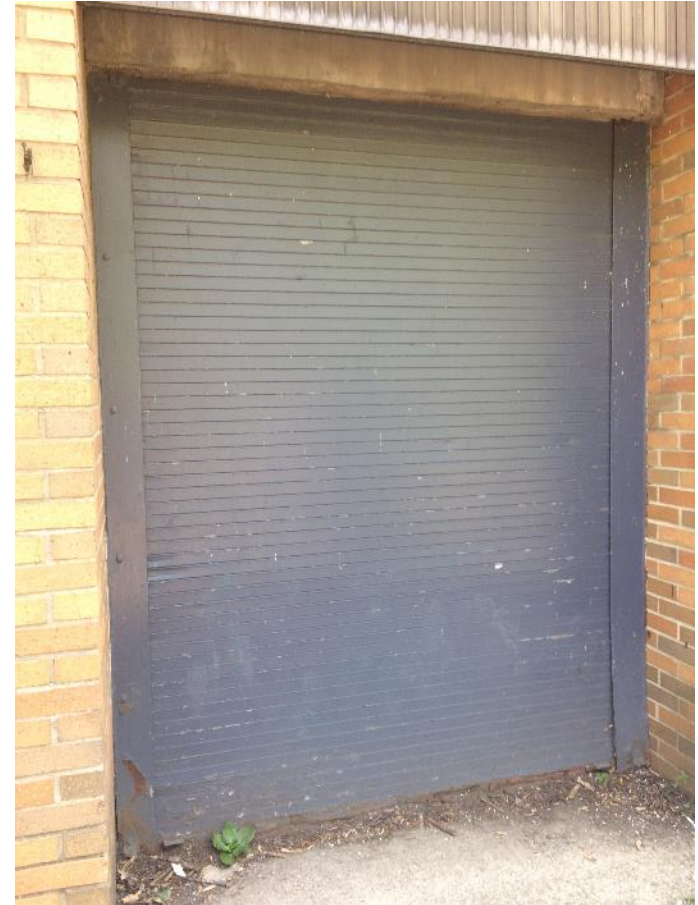
Exterior doors in poor condition
