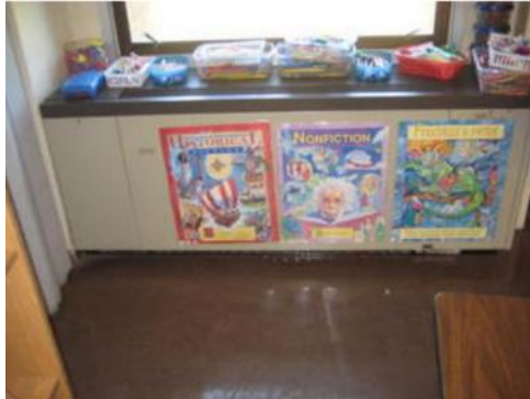
HVAC system does not provide 15 CFM fresh air per OBC
