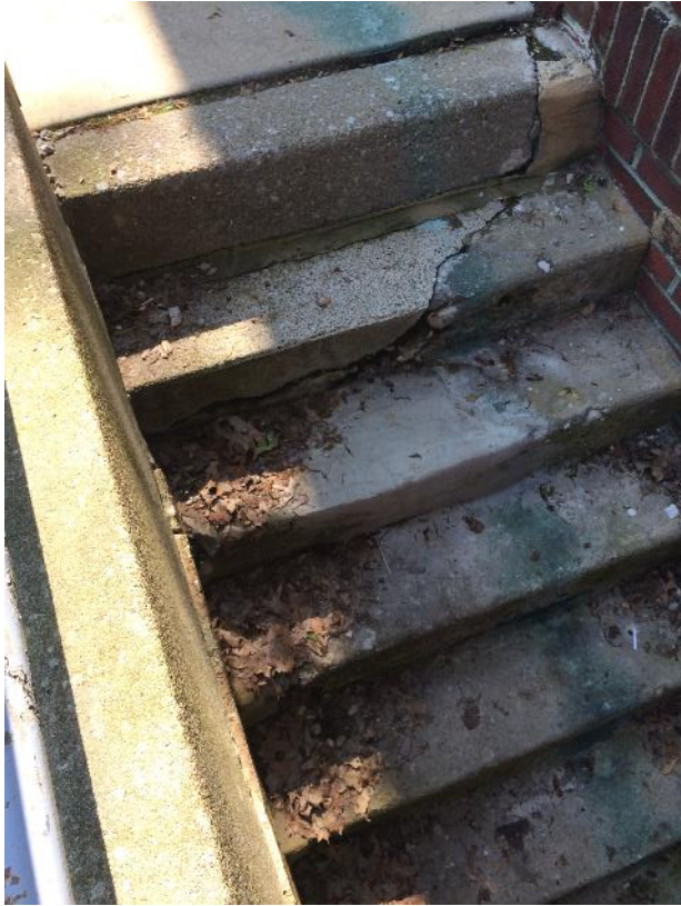
Concrete steps deteriorating
