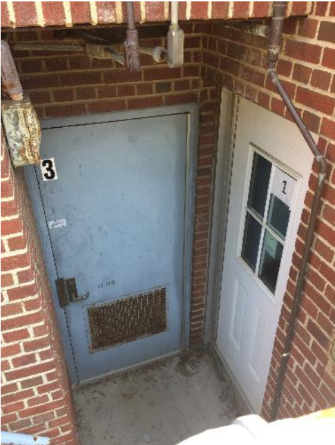
Exterior doors in worn out condition
