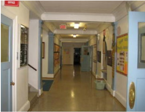
General Finishes in Worn condition
