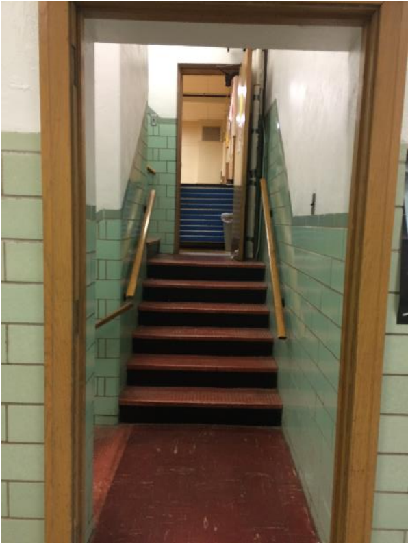
ADA barriers with multiple stories and level changes
