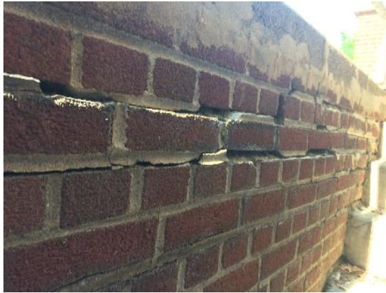
Retaining wall deteriorating
